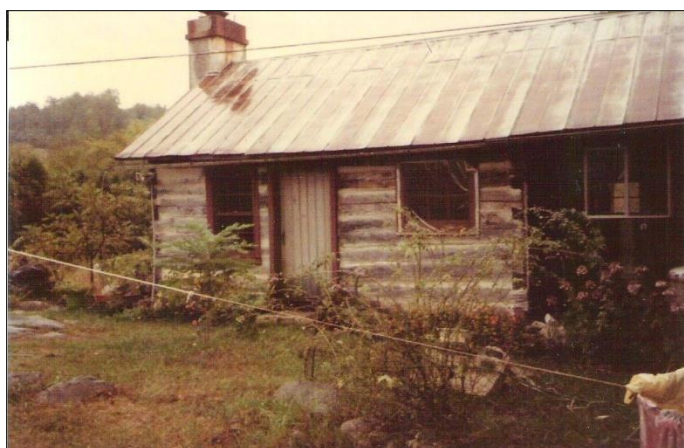
Back side of kitchen—before restoration. Photo courtesy of A.J. and Opal Frances Vaughan family, 1985.
